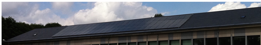
Plate 3. Solar panels on the school roof
